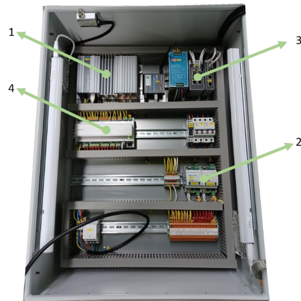
Figure 1: Electrical panel of the QEIR supervisor
