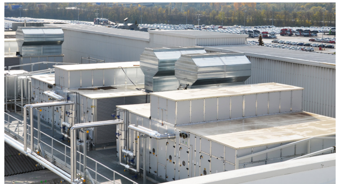
Roof-installed AHUs with ZerAx® axial fan
