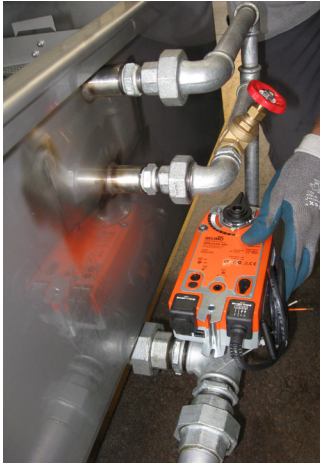
i) Mount a part of drain circuit primary tank (with bleed-off tank)
