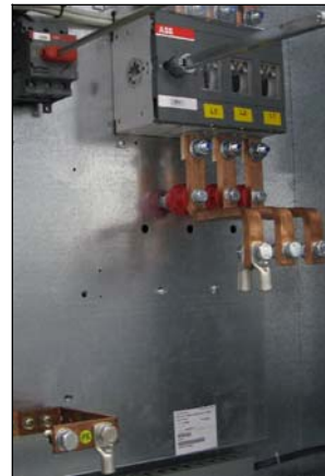
Fig. e - Example of connection with the disconnecting switch with 2 cable terminals and ground bar.
